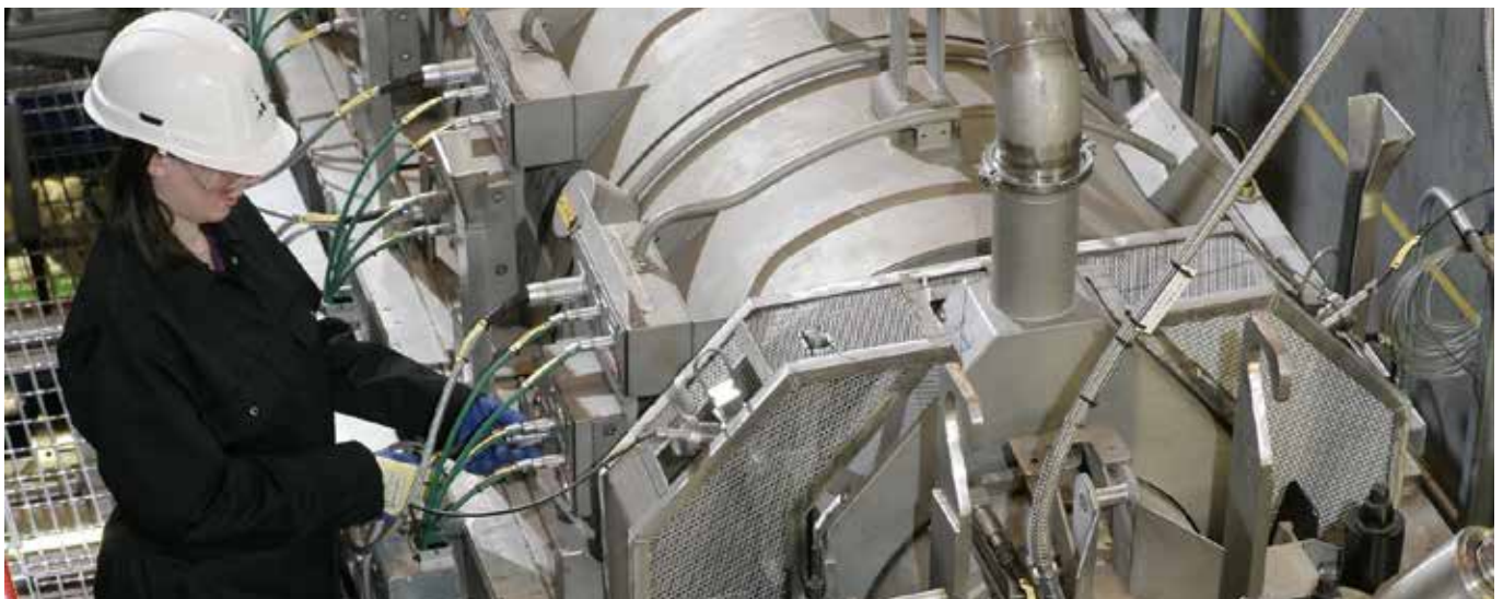
Figure 1: NNL's Vitrification Test Rig supports the UK HLW Waste Vitrification Plant at Sellafield
